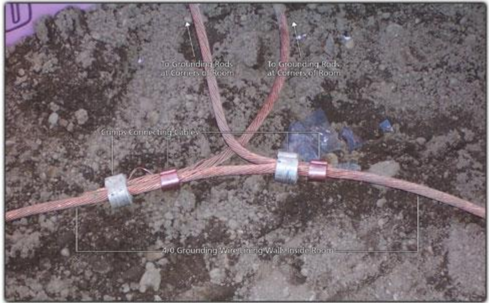
Figure 11. Cables connecting room grounding wire to grounding rods at corners of room
