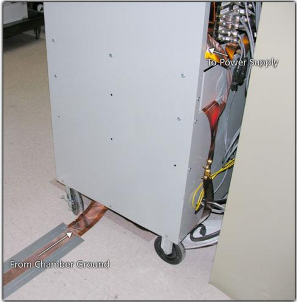
Figure 7. Copper ground strap leading to the power supply from the vacuum chamber
